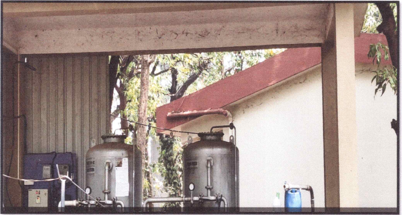
WATER PURIFICATION PLANT
