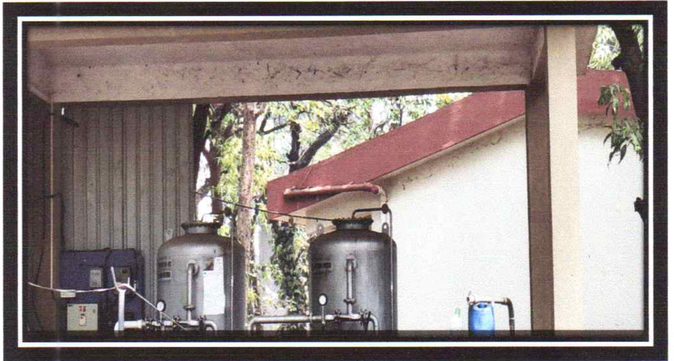
WATER PURIFICATION PLANT
